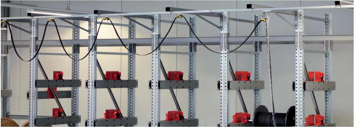
Fig.17 Cable trailing system for rack mounting
